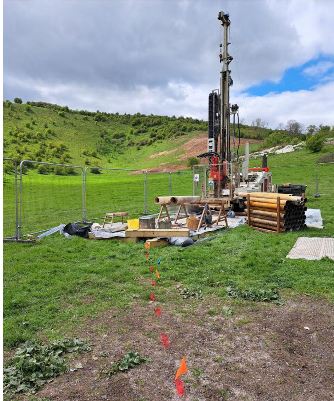
What the drilling rig looks like which you may see in the village
